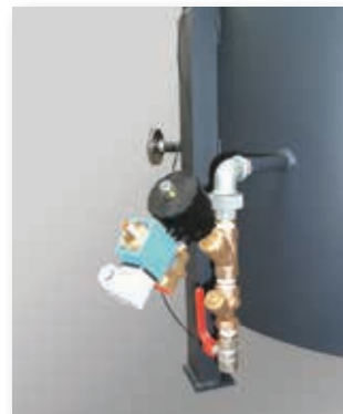
■ Cooling water inlet group
